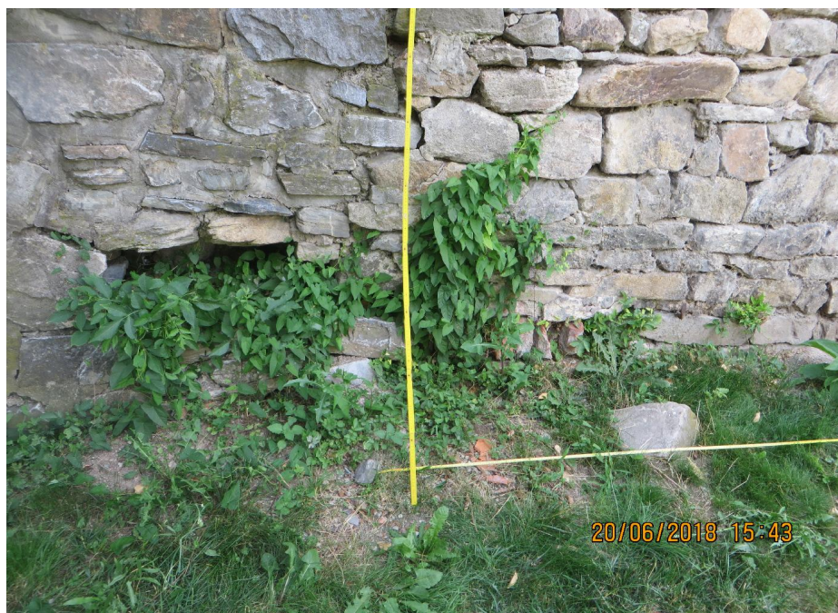
Obr. 20 Zed' Z7 - detail poruchy X5
