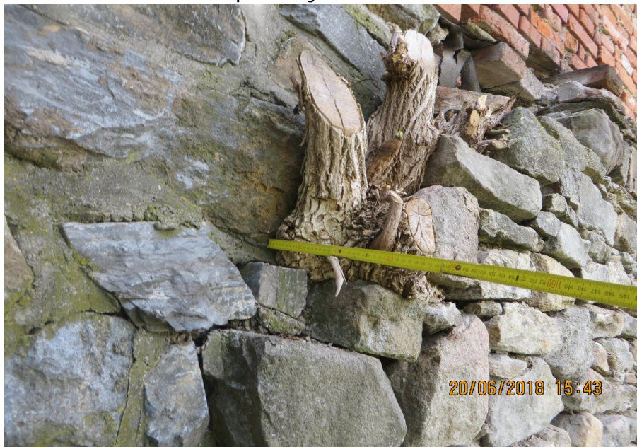
Obr. 19 Zed' Z7 - detail poruchy X4
